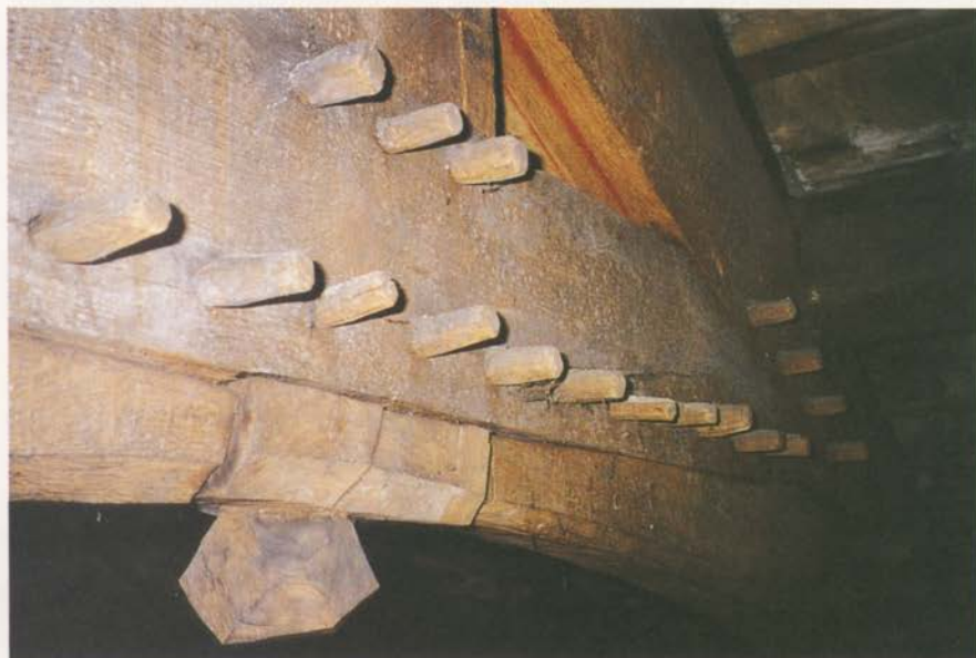
Milton House. The impressive arch-braced collar-beam truss shown here was intended to be seen although it is now hidden in the roof space of the house. The red lines created by the carpenter to mark out his work nearly 400 years ago remain clearly visible.
