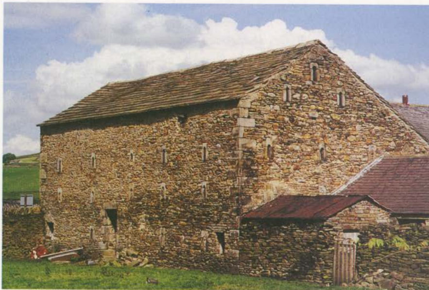
Pear Tree Farm barn and the adjacent garth. Before 1800 much of the land between Main Street and Back Lane would have been occupied by farm buildings and 'green' garths. These are now the only ones which remain part of a working farm.
